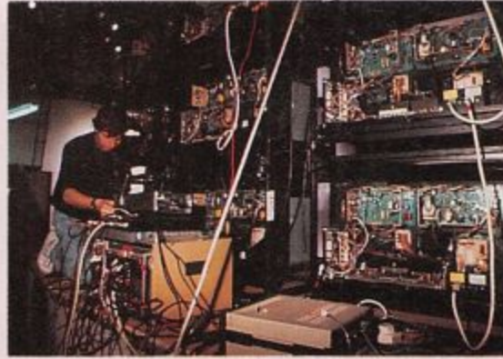
Creating virtual worlds is not for those who find wiring a plug a bit tricky, as this maze of wires and cables behind the glossy facade of the set indicates.
