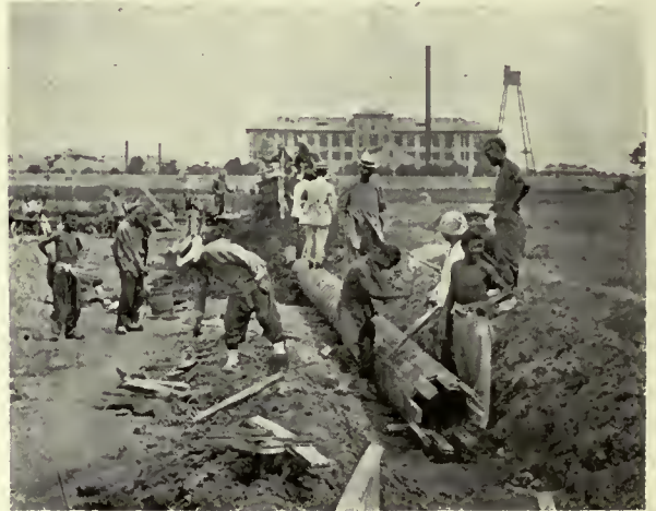
THE SCENE OF LAYING THE COMPANY'S WOODEN PIPES IN THE PEKING MINT.
